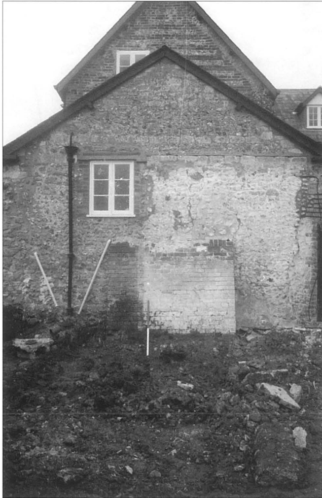
Figure 9: The east elevation of Woolcombe farmhouse in 1997 showing the ground floor byre wall. The white-painted area to the right of the downpipe and window represents the area adjoined by the former bottling plant. This part of the wall seems to have been made good and it is supported by a brick buttress (Bournemouth University)
