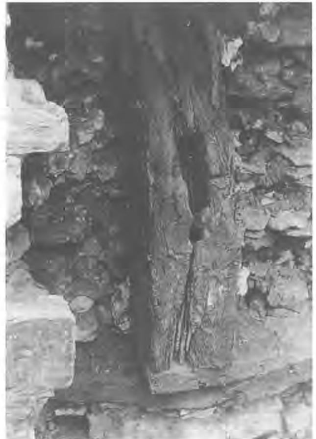
Figure 8. Hall House, Newland. Exposed base of cruck o / showing wall-post mortise with square hole below it.
