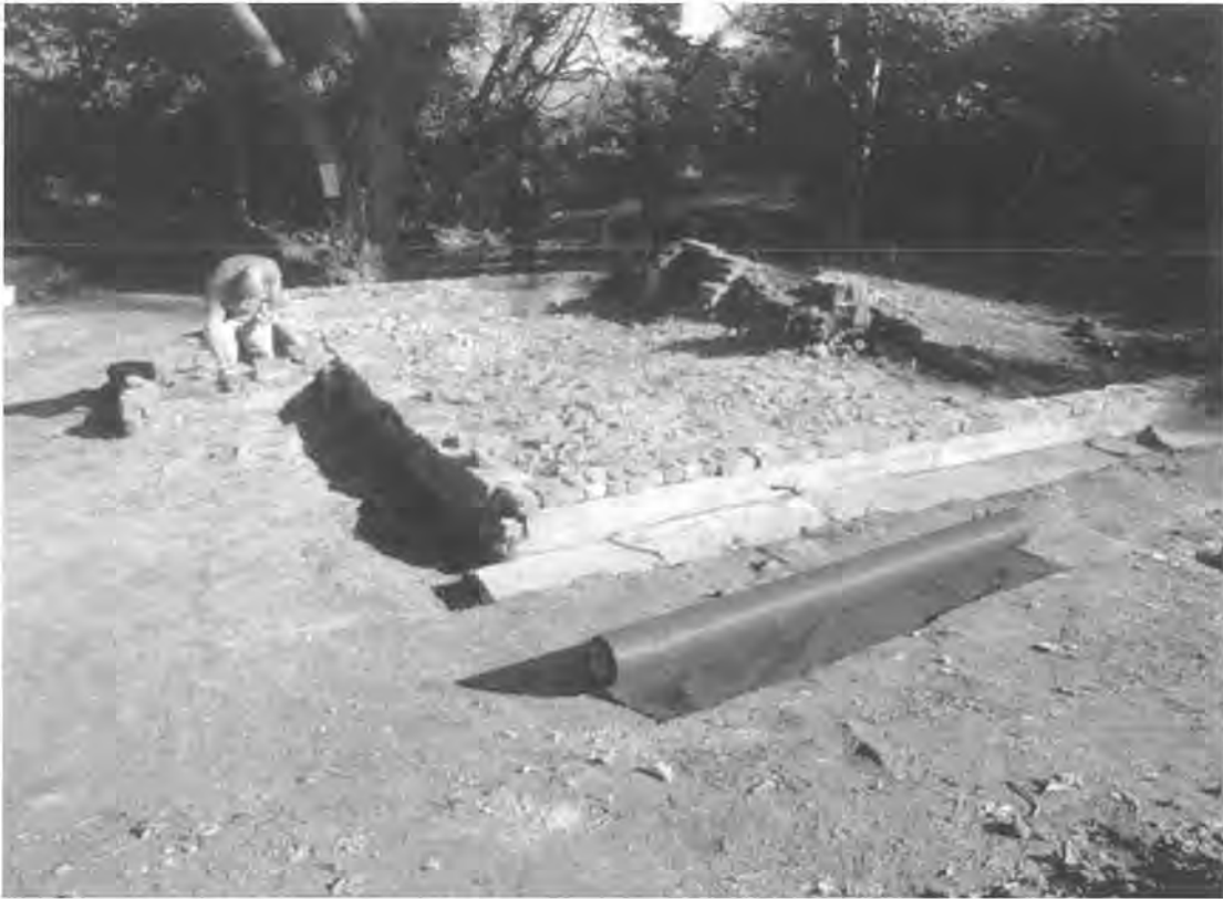
Figure 7: Raising the walls with bricks before covering the site with terram and topsoil. Line of flagstones abutting the back south wall of 1 Maryland
