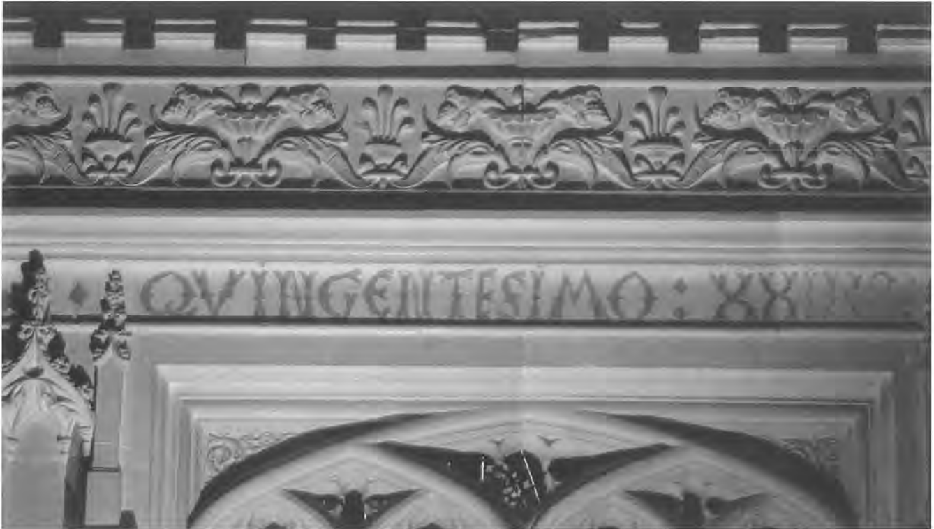
Figure 3: Christchurch Priory: Draper chapel showing the stringcourse with inscription, frieze, and cornice. (Photograph: Nicholas Riall)
