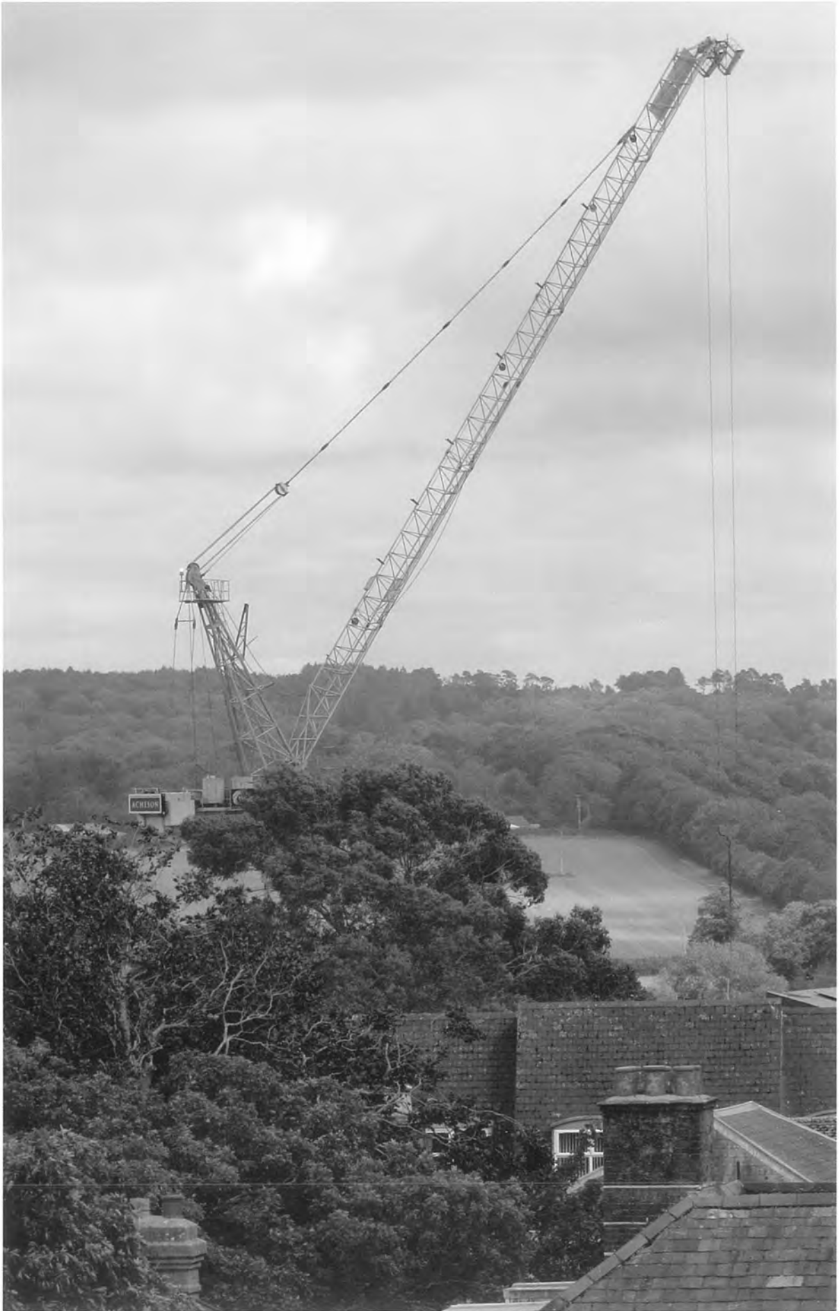
The tower crane used to construct the new Dorset Museum galleries looms over Dorchester. © DNHAS
