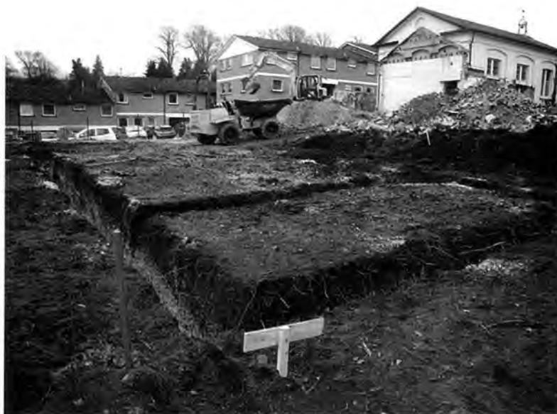
Figure 2 Site viewed from the north-west, with the footings for the new building in the foreground and the (former Grove) school building behind, top right.
