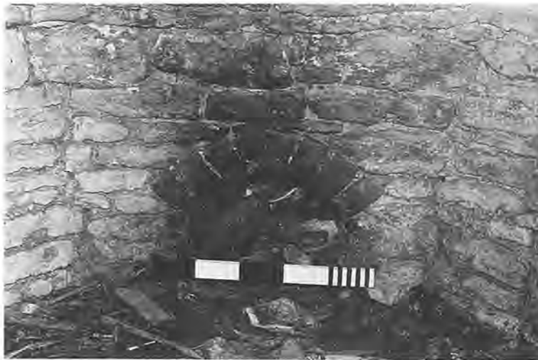
Plate 7. Brick-arched draw-hole at Downs Lane limekiln, Yetminster. July 1993. Scale: 0.5 metre.
