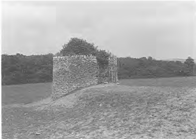
Plate 3. Whitmore Coppice limekiln at Langton Herring from the south, showing the retaining wall (restored) around the kiln head and pot. June 1993.
