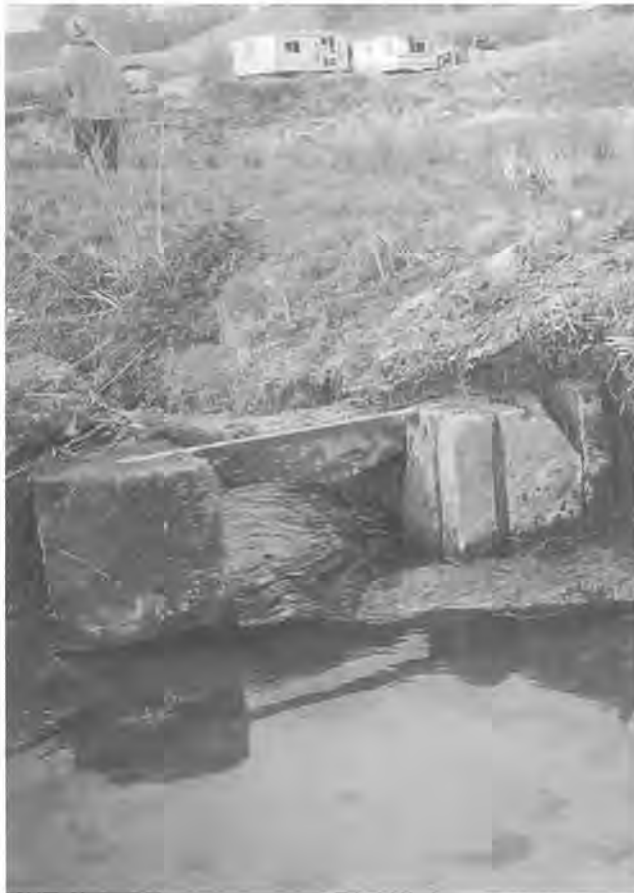
Plate 2 Sluice No. 2 from south-east side, showing remains of sluice and grooves for hatch.
